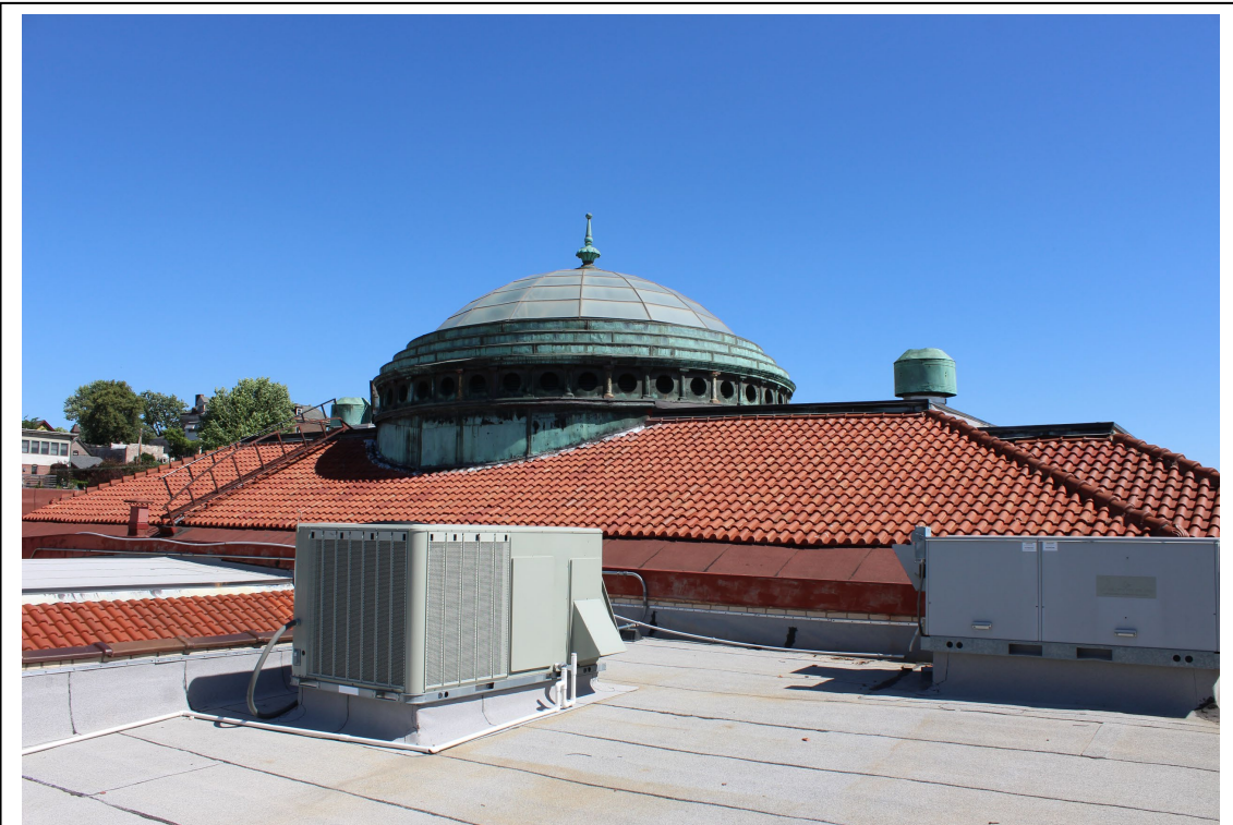
The roof and dome of the library with the roof of the 1916 addition in the foreground.
