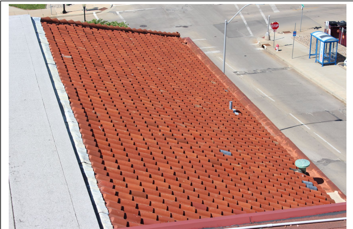
Detail of clay tiles on the rear ell with metal replacing missing tiles.
