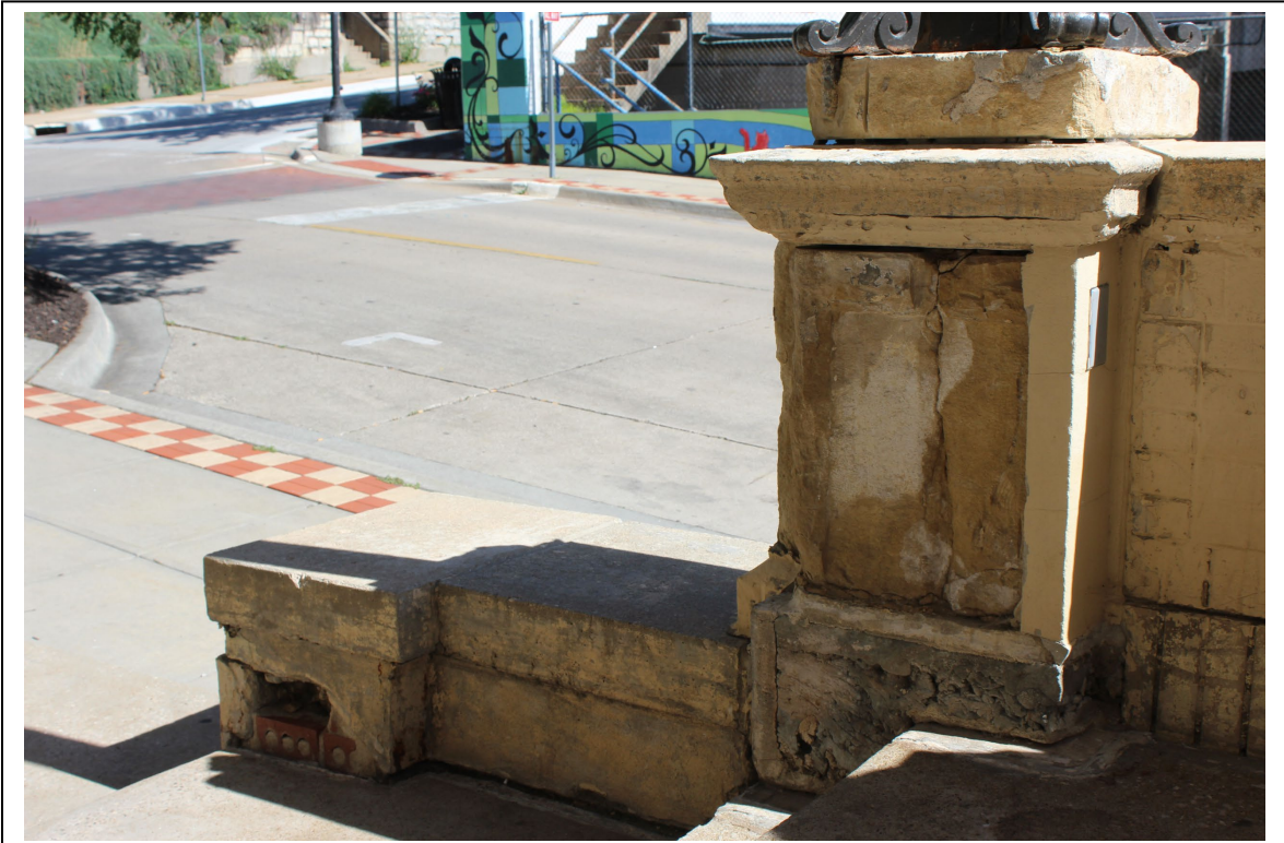
Detail of masonry deterioration at entry stair.
