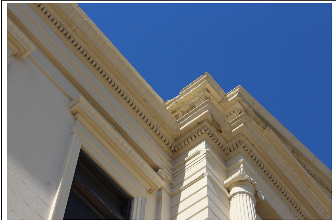
Detail of the deterioration of the cornice on the south elevation.
